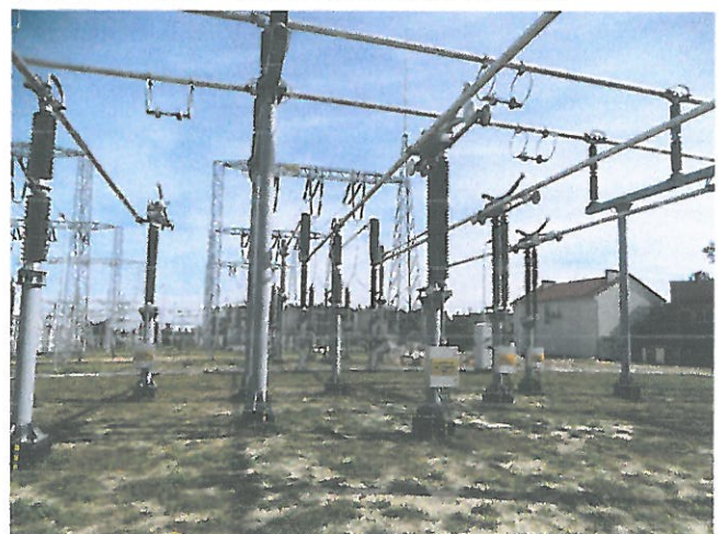
Pole 220 kV – Autotransformator AT1
