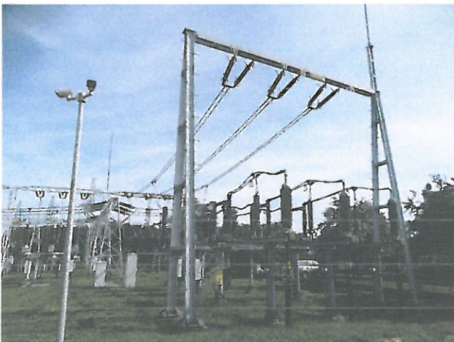
Pole 110 kV – autotransformator AT3
