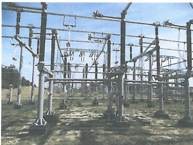
Pole 220 kV – Autotransformator AT2
